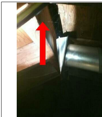
Exhaust vent should extend through roof.
